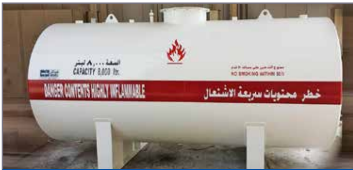
8,000L DIESEL STORAGE TANK
